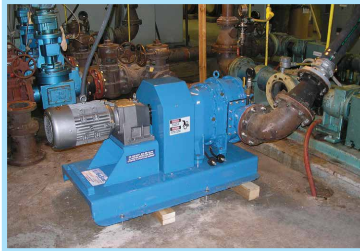
This 10-horsepower LobePro SL-133 was rebuilt fifteen months after installation in the wastewater treatment plant
