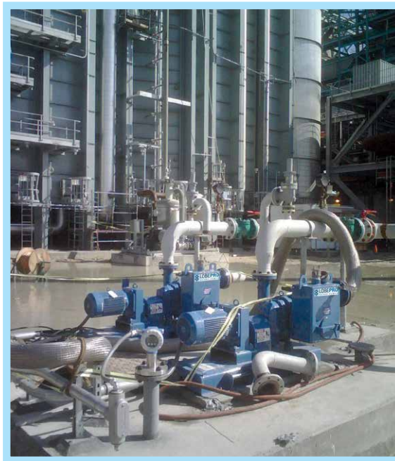
LobePro pumps were used for an oily water sump transfer application
